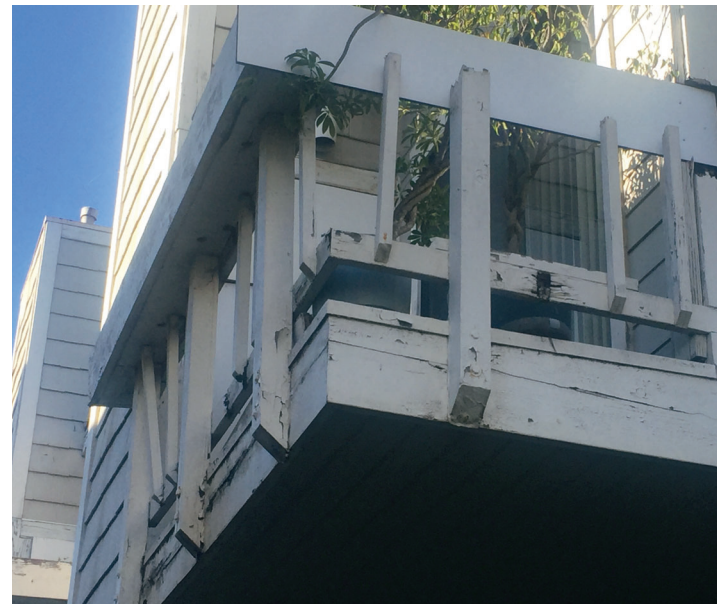
Figure 4: Dry rot and weakened balcony rails that will fall anytime.
