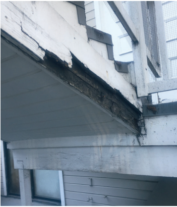
Figure 5: Walkway with extensive dry rot damage.
