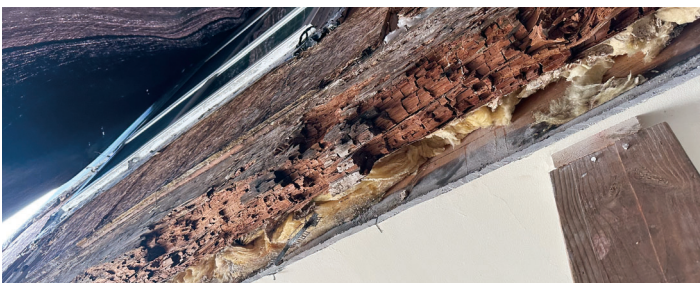
Figure 3: Termite and dry rot damage
