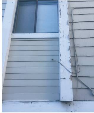
Figure 6: Exterior dry rot that signals possible wall damage, but we don't know until this is opened.
