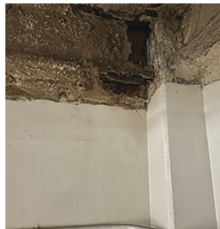
Figure 11 Corrosion effects on steel frame moment connection in parking structure.
