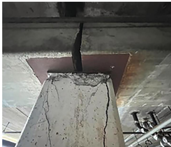
Figure 13 Subterranean parking column cracking with no seismic lateral connection on the beams.
